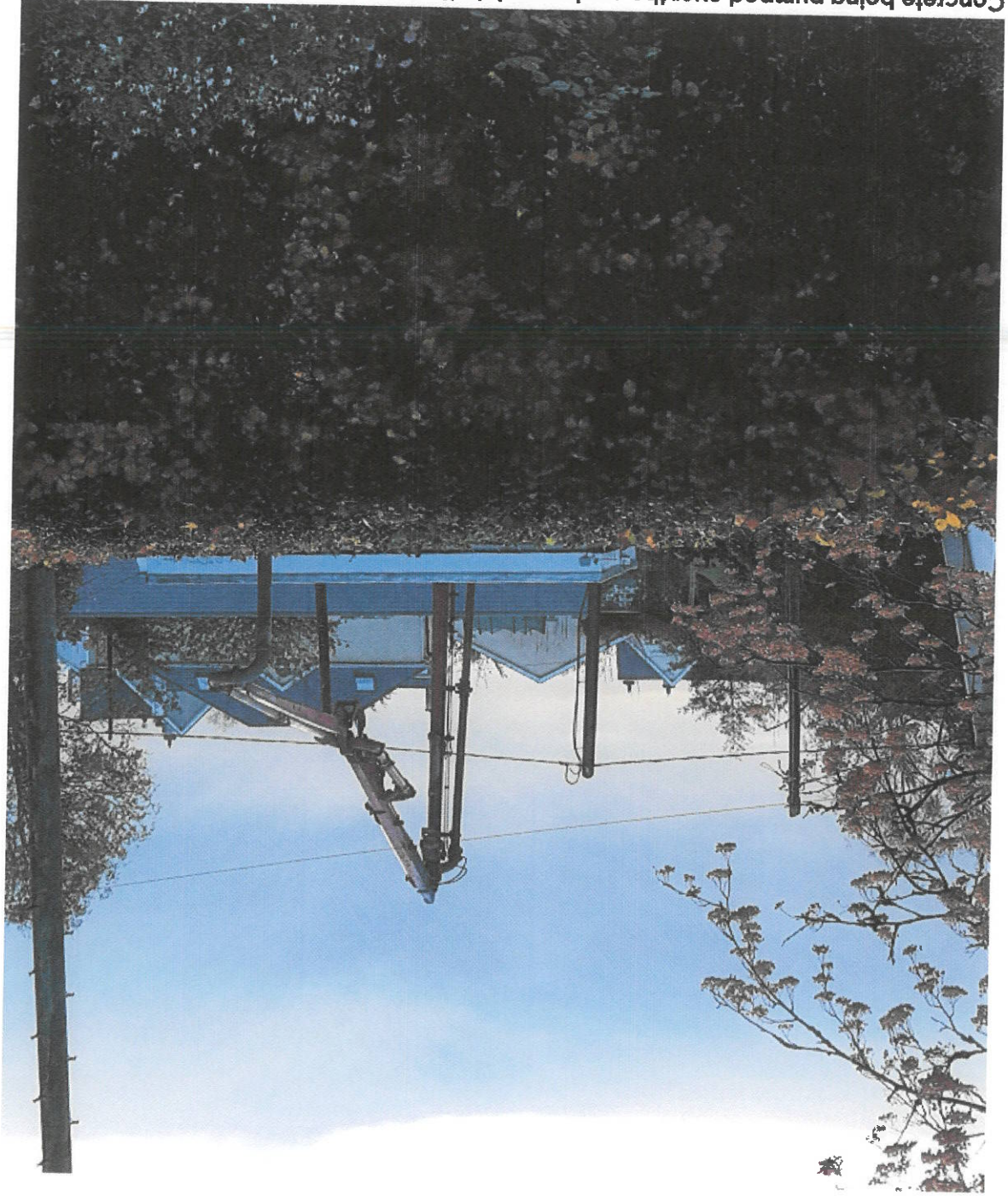
Concrete being pumped over the exchange into the excavation at 8.30am, 15 November 2021
