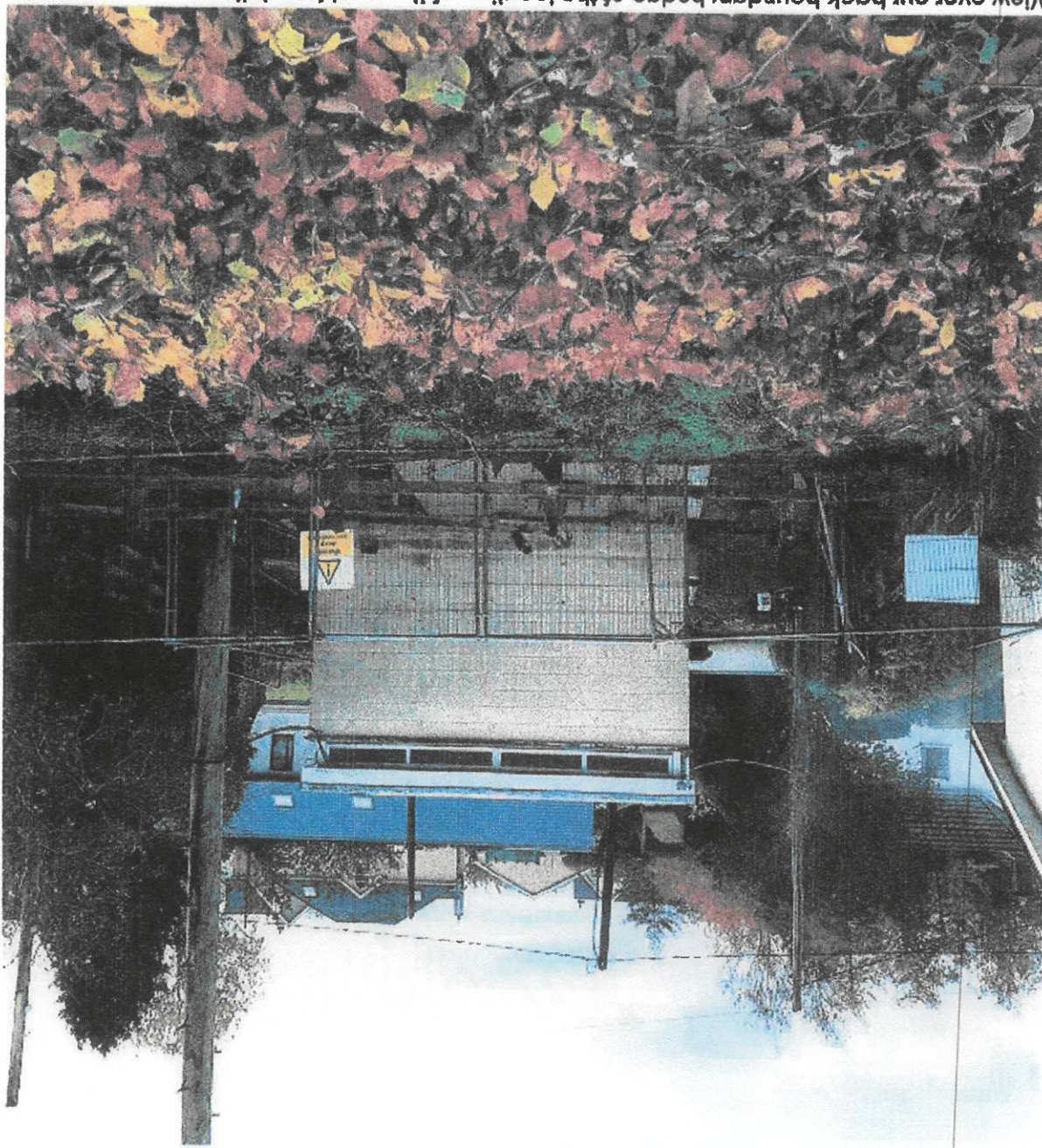
View over our back boundary hedge of the location of the mast foundation
